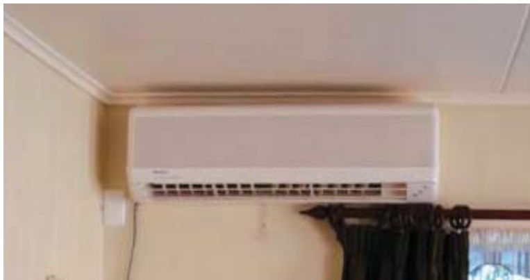
Rough installation unit too close to the ceiling.
